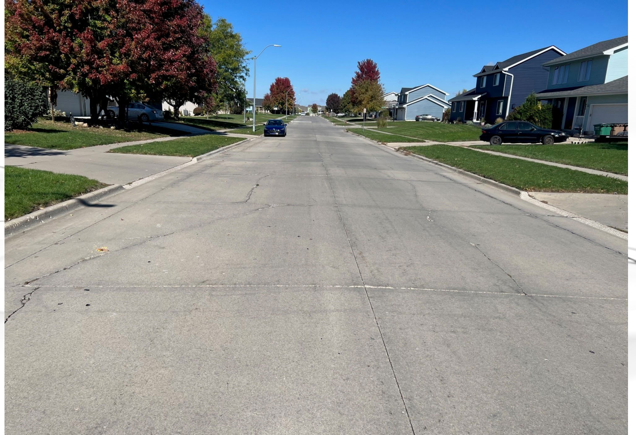
Poor jointing and early 'D' Cracking
