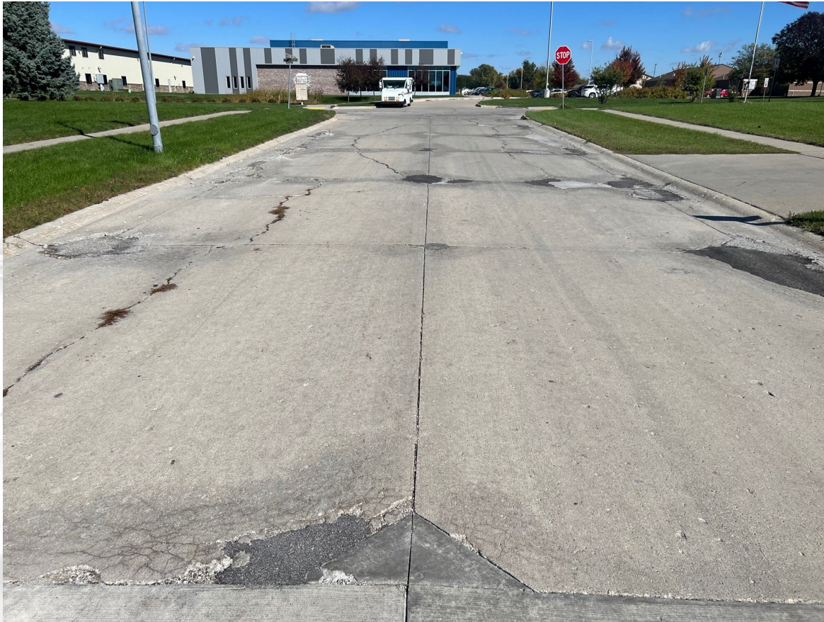
Poor jointing and advanced 'D' Cracking
