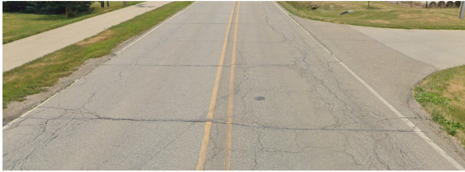
FIGURE 17: EXAMPLE OF “FAIR” CONDITION (ACC) – 2ND STREET This picture of 2 nd St near Snyder St is an example of an ACC pavement that was rated as 45/100 which would be considered “Fair.” It has some transverse and alligator cracking.
