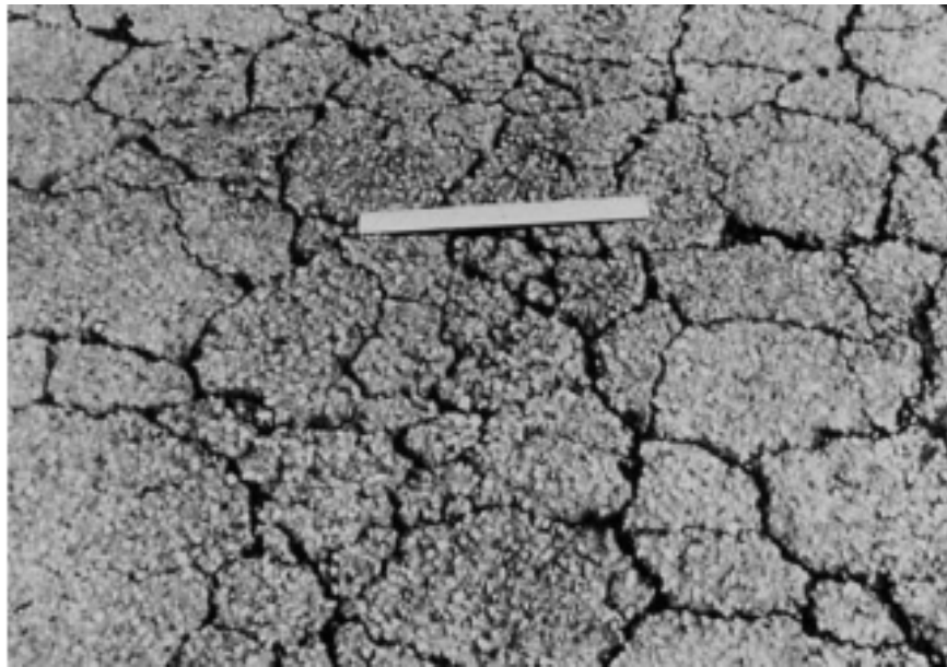
FIGURE 5: EXAMPLE OF ALLIGATOR CRACKING (ASTM)
