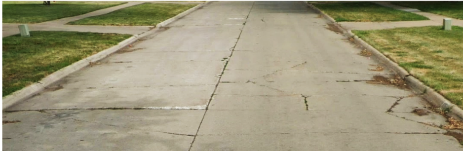
FIGURE 18: EXAMPLE OF “POOR” CONDITION (PCC) – 4TH STREET NE This image shows a PCC street whose pavement is rated as 33/100. 4 th St is considered to be in “Poor” condition due to rideability issues caused by settlement and cracking.
