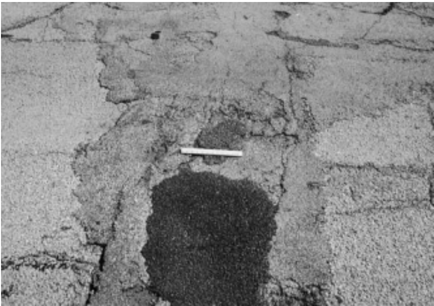
FIGURE 9: EXAMPLE OF PATCHING (ASTM)
