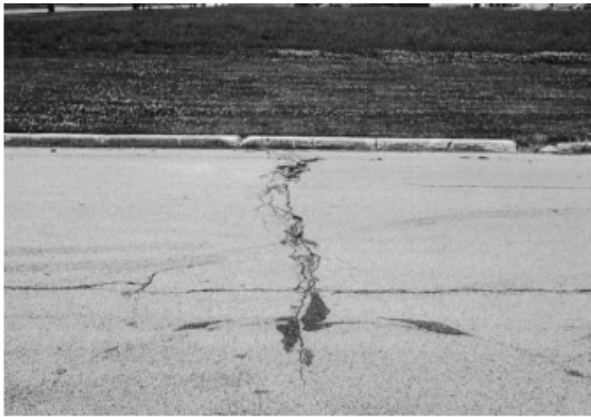
FIGURE 8: EXAMPLE OF TRANSVERSE CRACK (ASTM)
