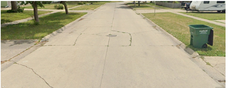
FIGURE 16: EXAMPLE OF “FAIR” CONDITION (PCC) –ALPHA STREET This image of Alphas St is an example of PCC pavement in “Fair” condition, with a PCI of 59/100. There are very noticeable distresses but only on a handful of panels.
