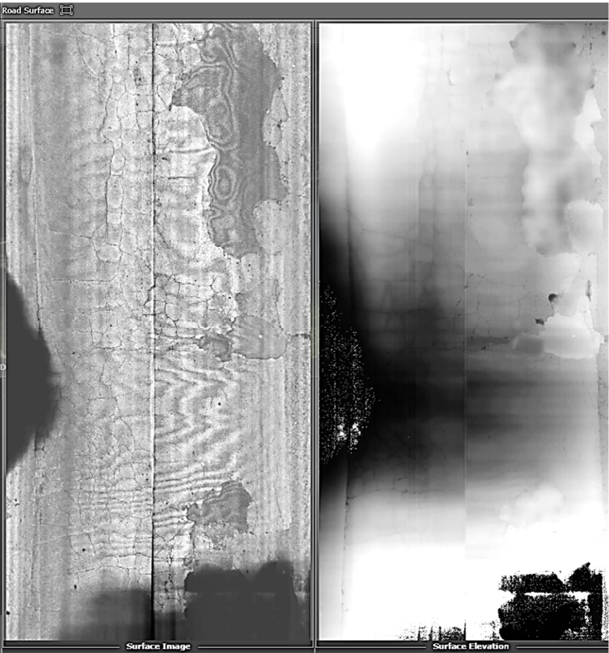
FIGURE 45: UNACCOUNTED FOR FAILURE
