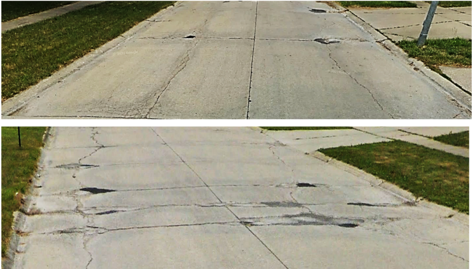
FIGURE 22: EXAMPLE OF “VERY POOR” CONDITION (PCC) – 10TH STREET SE This image shows a PCC street whose pavement is rated as 11/100 and considered to be in “Very Poor” condition. 10 th St east of Lincoln Ct has point failures and significant cracking.
