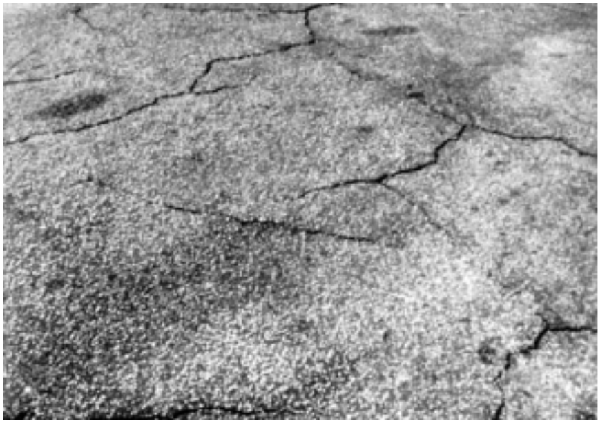
FIGURE 6: EXAMPLE OF BLOCK CRACKING (ASTM)
