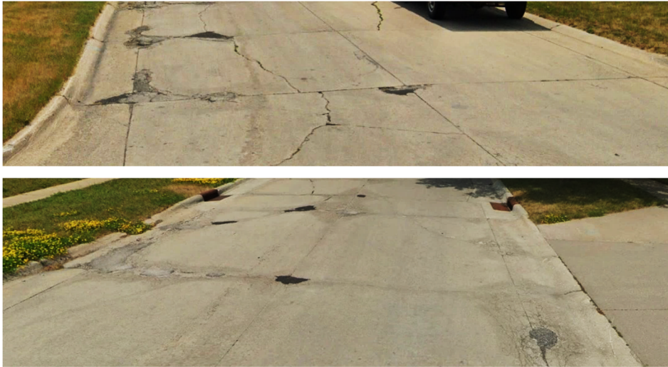
FIGURE 20: EXAMPLE OF “VERY POOR” CONDITION (PCC) – BRICK STREET SE This image is an example of a PCC pavement in “Very Poor” condition. Brick Street SE is considered one of the worst condition roads in the system due to widespread joint failure and many cracked panels.
