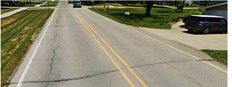
FIGURE 14: EXAMPLE OF “GOOD” CONDITION (HMA) – 2ND STREET SE This picture of 2 nd St between Blaine St and Deer Ridge Dr was rated as 66/100, which would be considered Good for an HMA pavement. Small transverse cracking and rutting is noticeable on this pavement.
