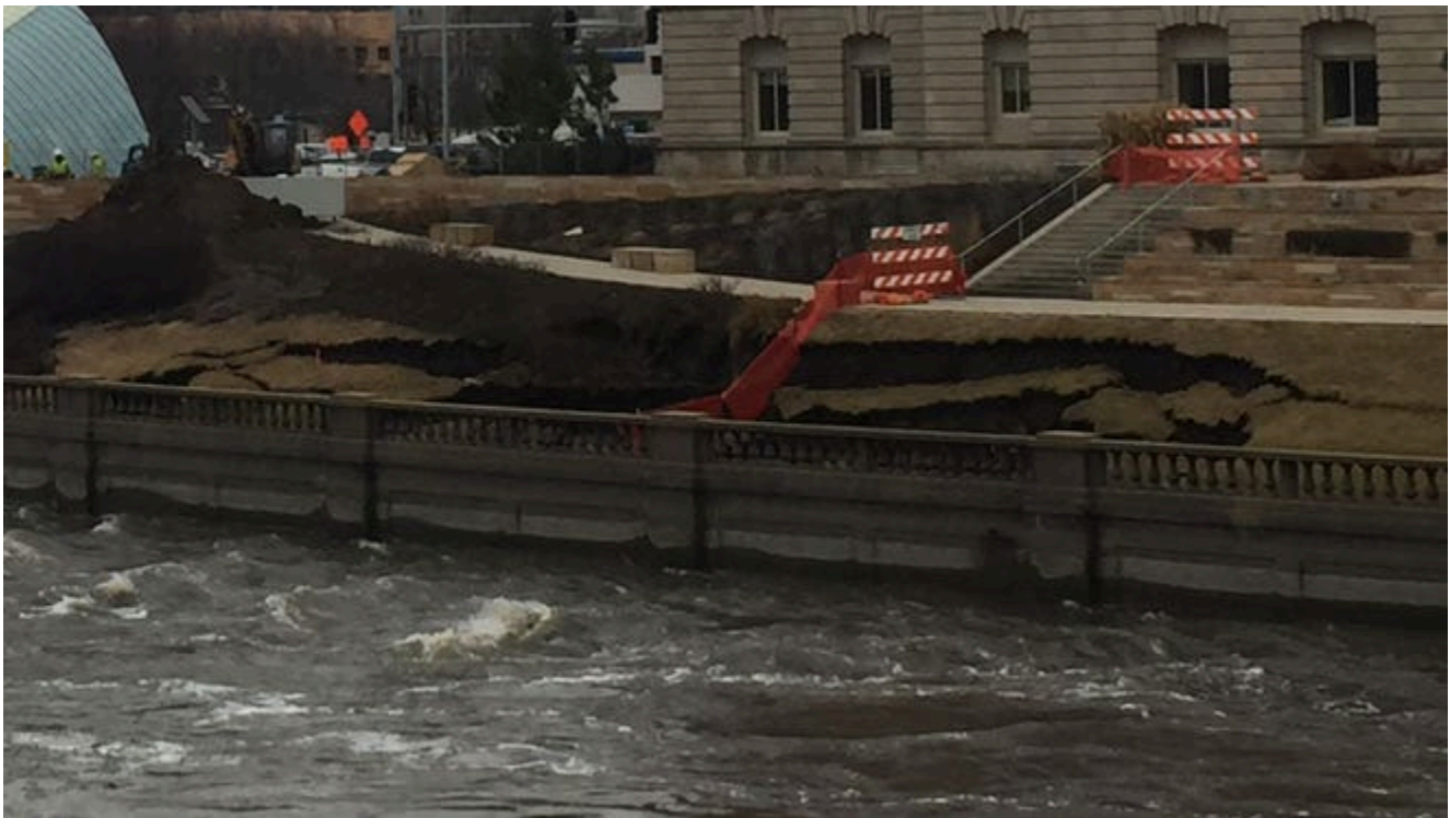
Figure 106. Landslide along the bank of the Des Moines River 2017
