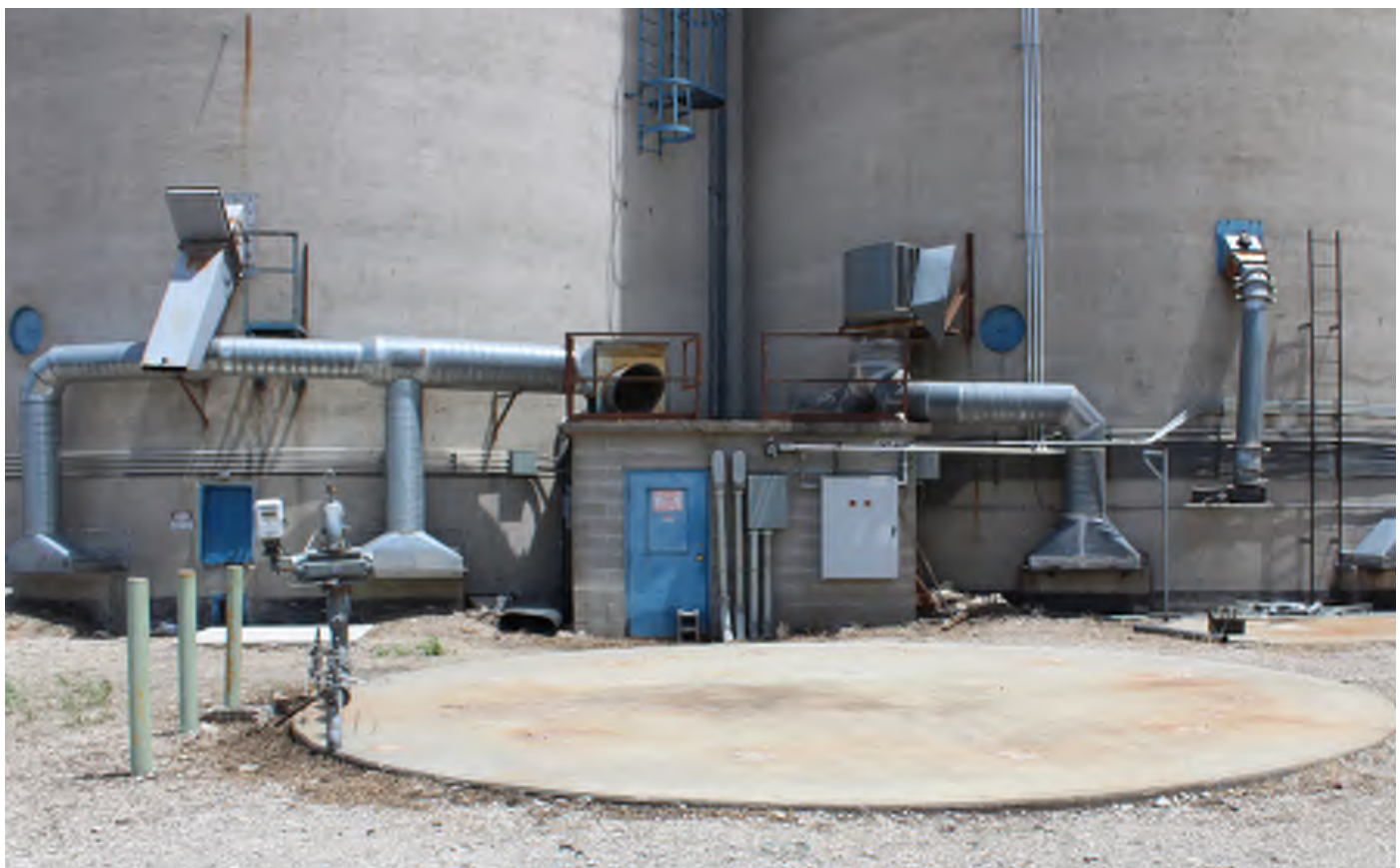
Electrical Room + Mechanical Ductwork
