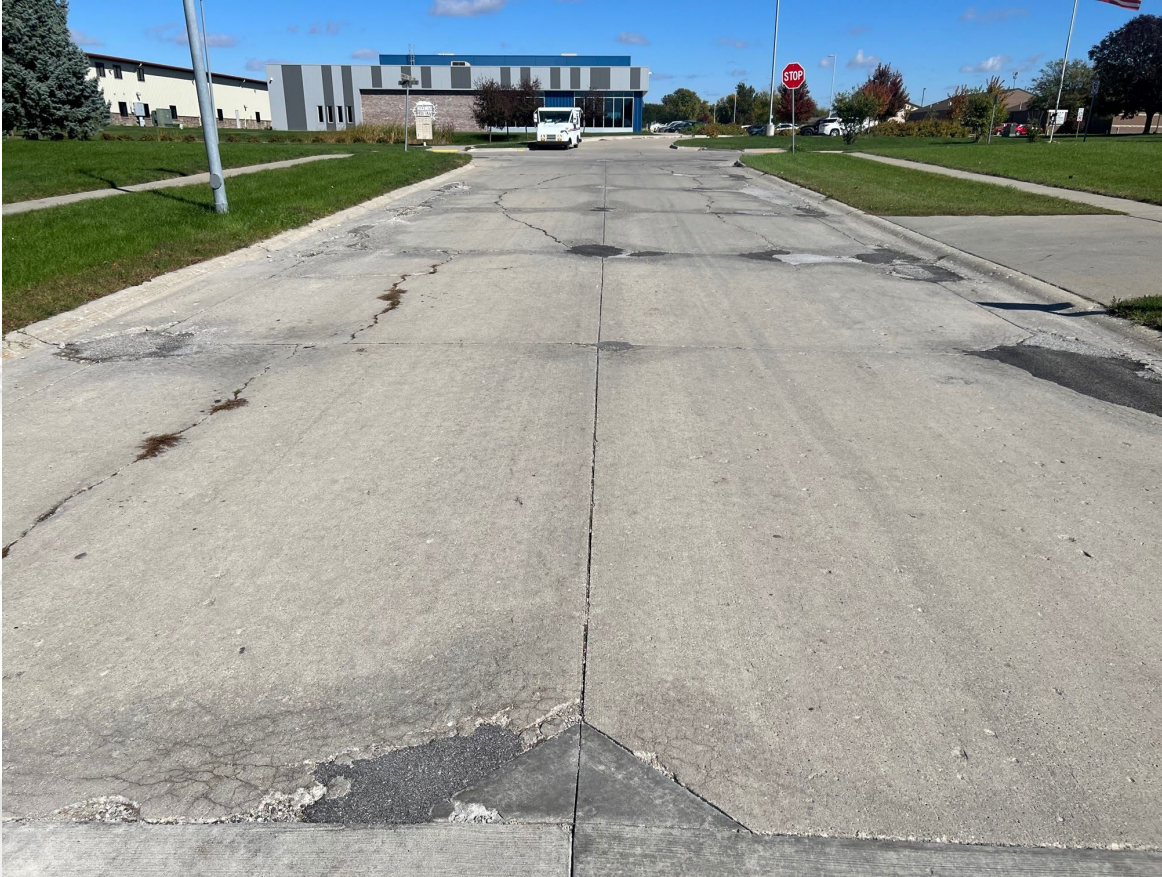
Poor jointing and advanced 'D' Cracking
